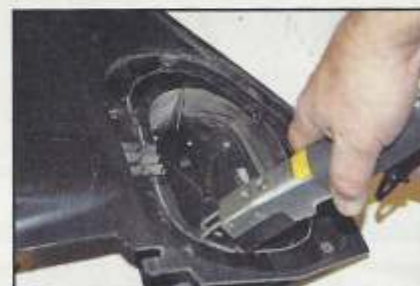
•After removing the passenger side kick panel, we used the template included with the kit to outline the cut for our new insert. We cut the opening using an air-powered body saw.
