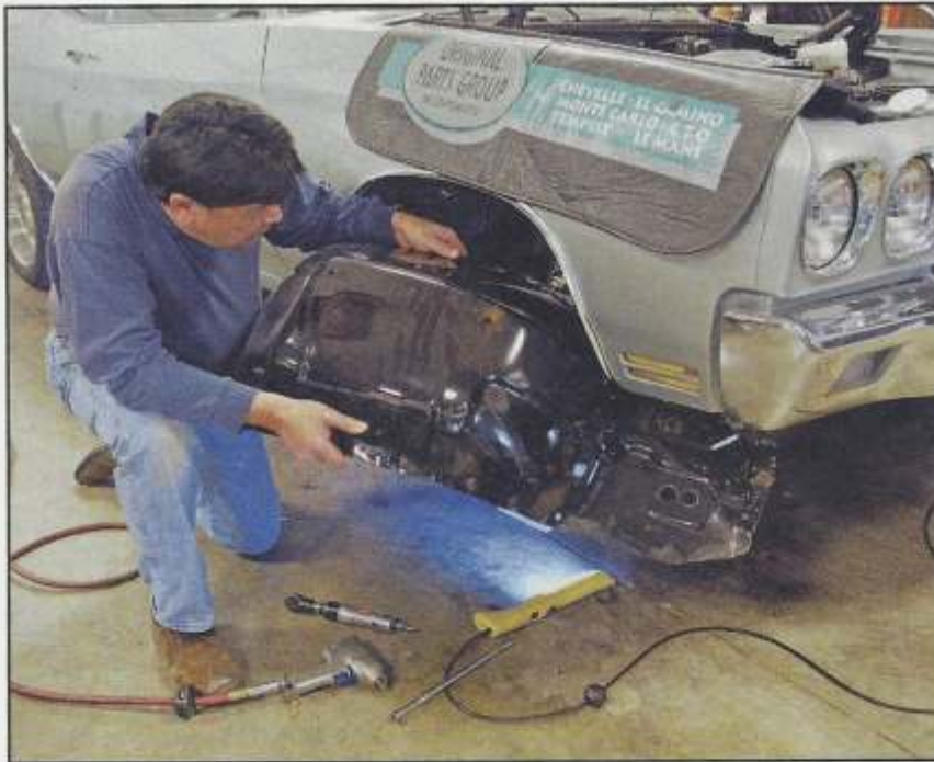
•To access the original heater assembly and provide room to route the new A/C hoses, we removed battery, battery tray, and the right, front inner fender.
