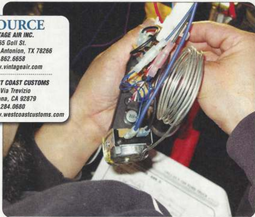
Mosco actually wanted to test the wiring on the controls in a position where he could easily get to it, so he connected all of the wires while the controls were still uninstalled.
