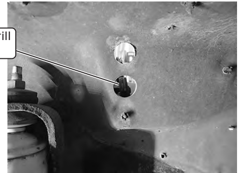
Wheel Well Side
